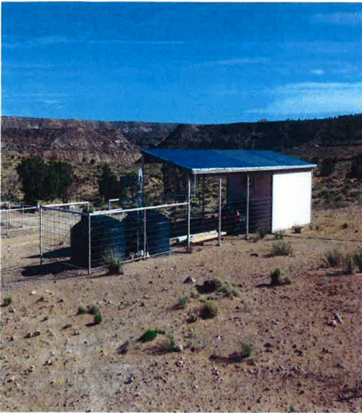
Rain harvester and tanks
